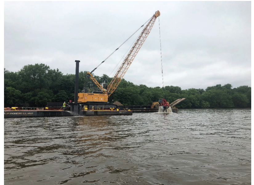
MVR MECHANICAL 19-25 SEP (289 UMR) 21-26 OCT (241 UMR)
